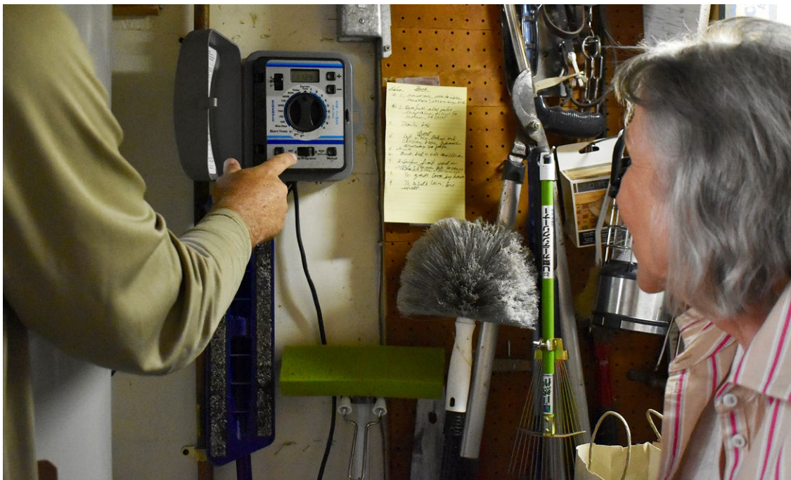
Irrigation frequency and run times are reviewed for each planting zone at the sprinkler irrigation controller. Photo: Rebbeca Ryan.
